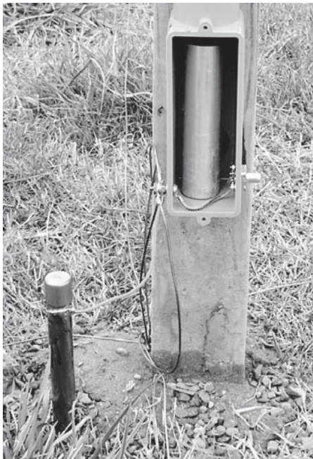
Figure 19 — You can see the ground rod and radial attachment for a vertical in this photo.
